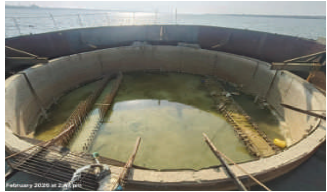
Fig. 5: Interior of the well cap enclosure (6 February 2026) showing the circular steining wall, exposed reinforcement dowels projecting from the cut base, and temporary water pooling in the lower levels following a minor steining defect. The enclosure is being dewatered prior to resuming cutting operations.
