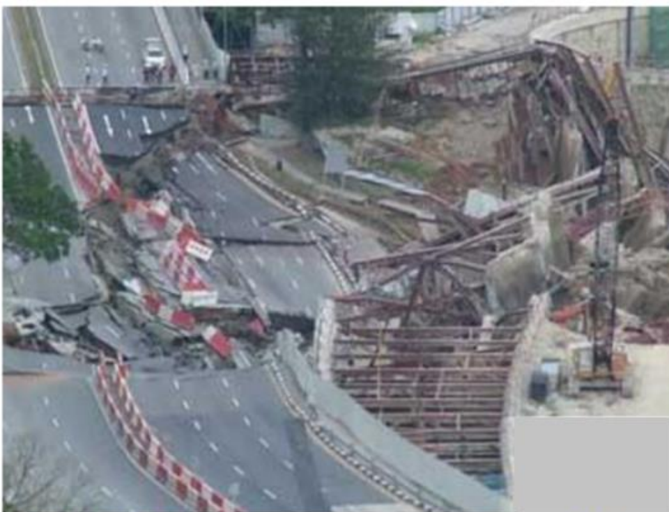
Nicoll Highway collapse, Singapore August 2004 Deep excavation under construction tunnel
