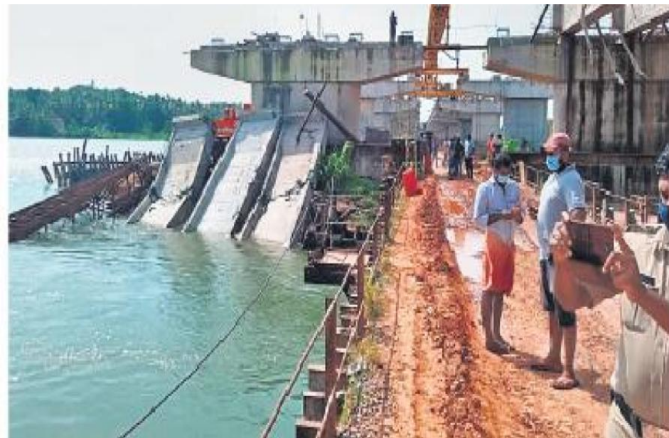
3 beams of bridge under construction in Thalassery(Kerala) collapse.....August 26, 2020.
