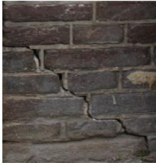
Cracks due to shear deformation
