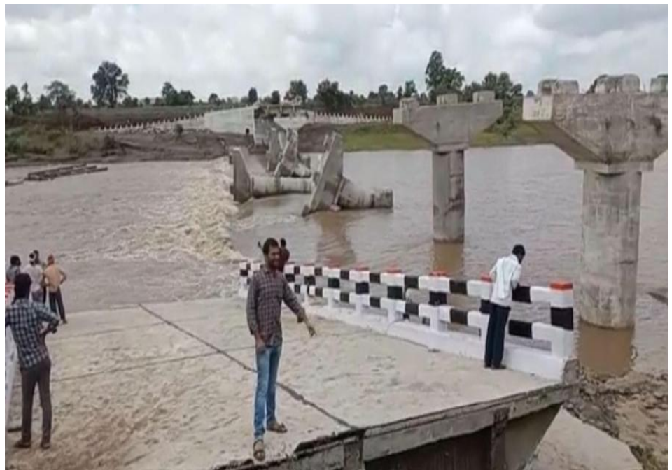
New bridge, collapsed MP, August 30, 2020
