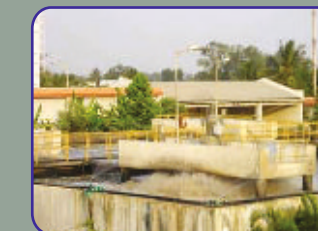
2004 - Waste Water Treatment Plant, Mylasandra, Bangalore
