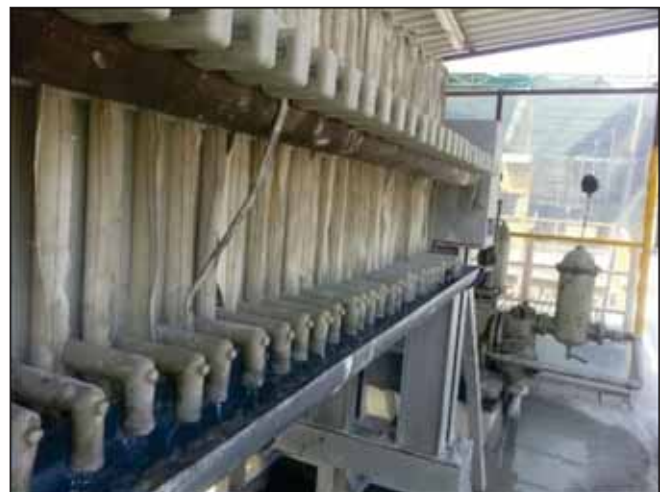
Fig 17 : Typical reclaimer set-up used in RMC plant for recovery of fine materials and wash water (above) and filter press system capable of delivering clean water and sludge cakes from wash water (bottom)
