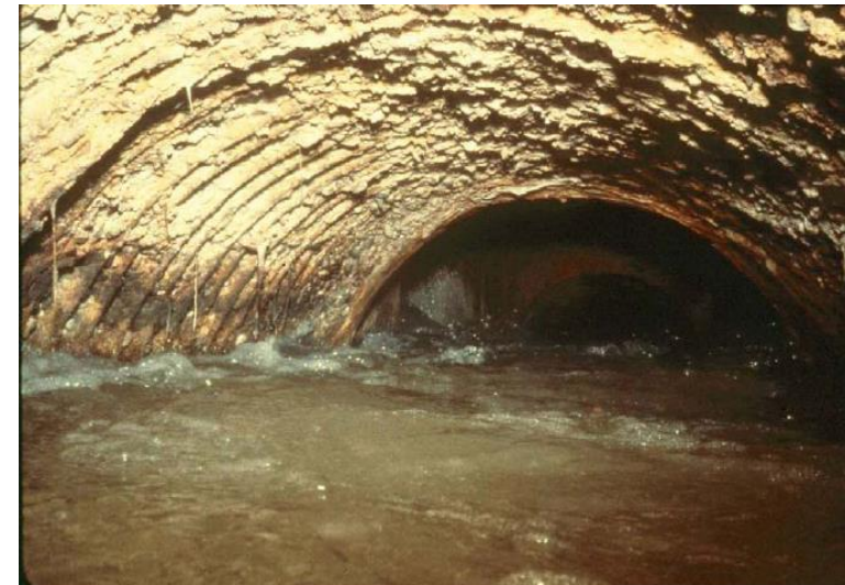
Figure A.4.2.2 Disintegration of sewer pipe by chemical attack due to H_2S .
