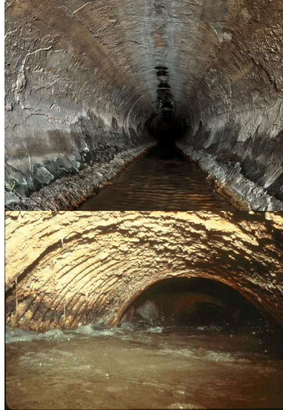
Figure A.4.2.2 Disintegration of sewer pipe by chemical attack due to H 2 S.
