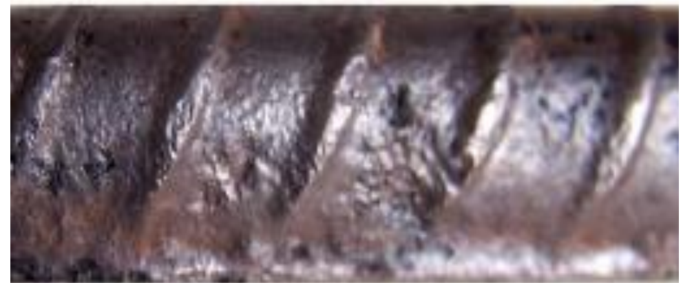
Corrosion of steel
