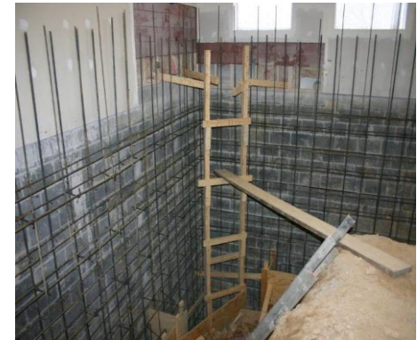
Improper construction methodology
