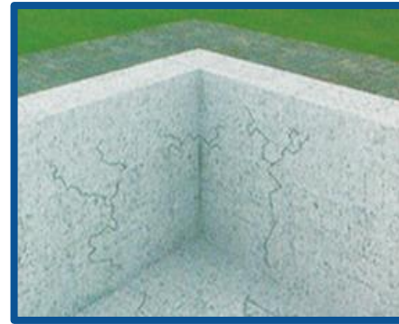
Water tank structure is not rigid hence makes it prone to water ingress when structure slightly moves
