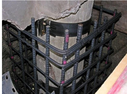
Defective structural design
