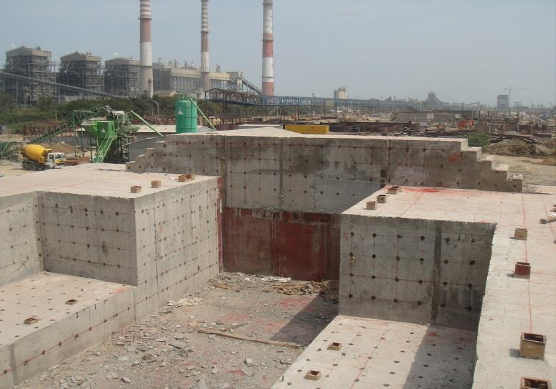
BHEL Thermal Power Project at Tuticorin, Tamilnadu
