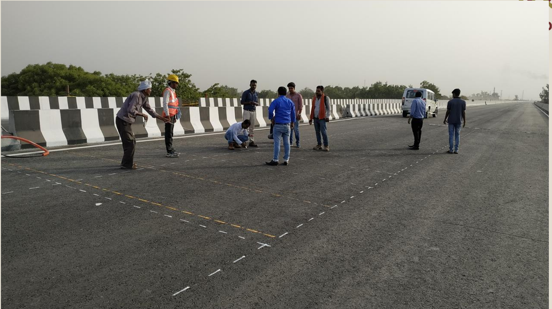
VIEW of tyre print marking on carriage way for carrying out load test
