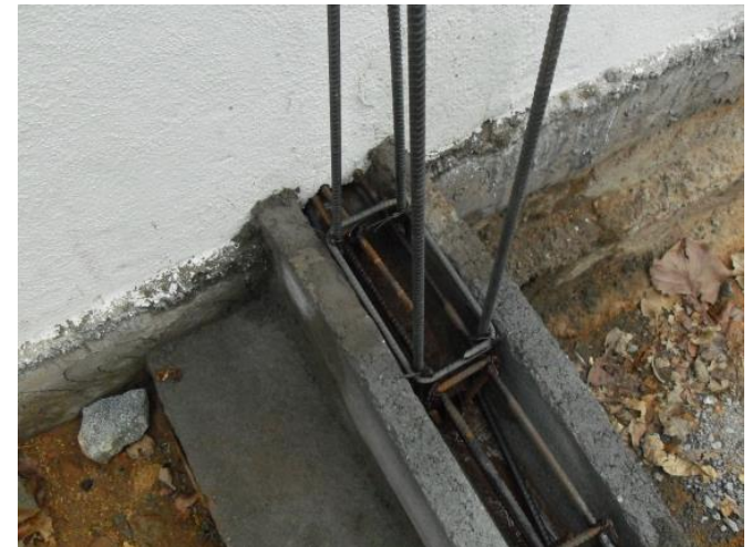
Pillar rods (if required) tied to the Plinth beam rods before casting plinth →
