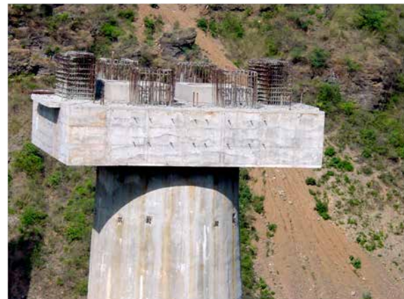
FIG. 22 PHOTO OF SEISMIC RESTRAINERS
