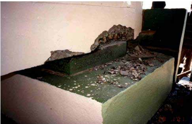
FIG. 1 DAMAGE AT BEARING LEVEL IN NEW SURAJBARI BRIDGE
