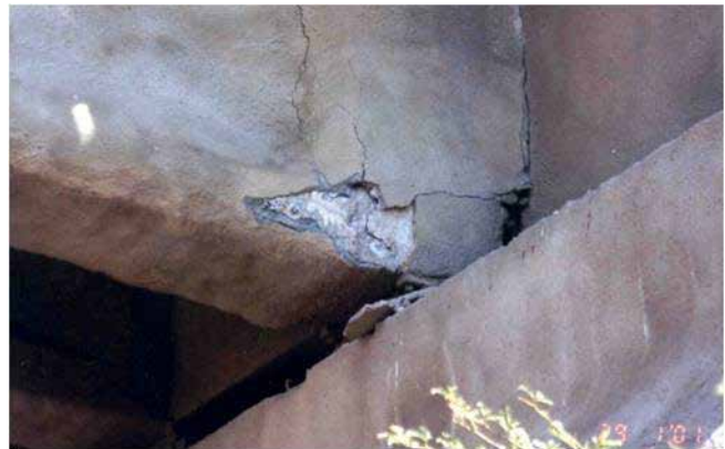
FIG. 2 MACCHU BRIDGE SUPERSTRUCTURE POUNDED THE DIRT WALL
