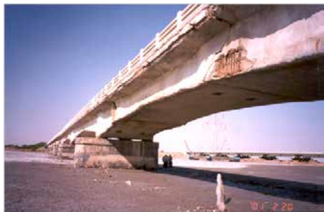
FIG. 4 SURAJBARI OLD BRIDGE HALF JOINT IN DISTRESS DUE TO VERTICAL AND HORIZONTAL SHAKING
