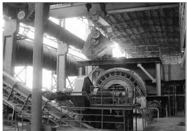
Fig 3: Slag Granulation Plant
