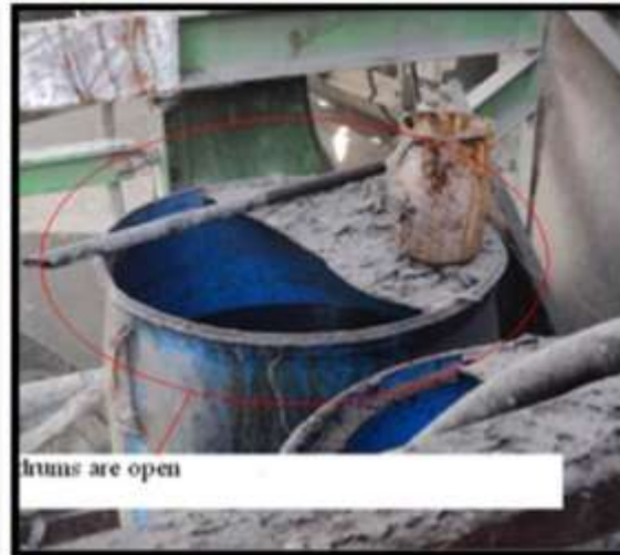
Highly incorrect method of pumping admixture with drum lid cut open
