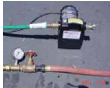
Fig. 17. Image of the hand held applicator and its position during the water test of the gutter area as well as the positioning of the spray rack system
