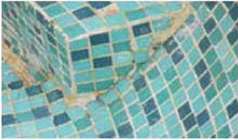
Fig. 14 Digital Image of leakage spot
