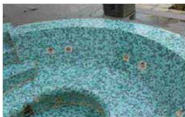
Fig. 11. Digital Image of leakage spot
