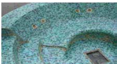
Fig. 11. Digital Image of leakage spot
